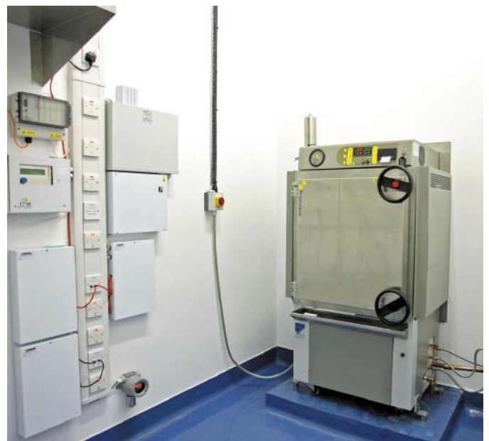
The service end showing the autoclave and water softener in-situ.
